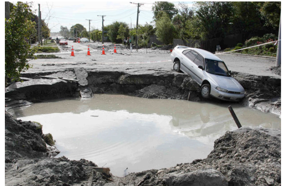
Roads were damaged in unpredictable ways.
