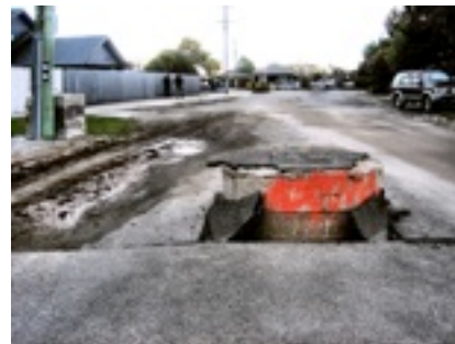
Liquefaction conceals a ruptured sewer line.
